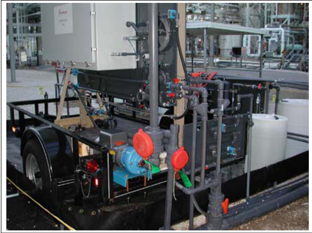
Figure 1: Field Test loop for exposure of Multielectrode Array Sensor Probe and Corrosion Coupons
